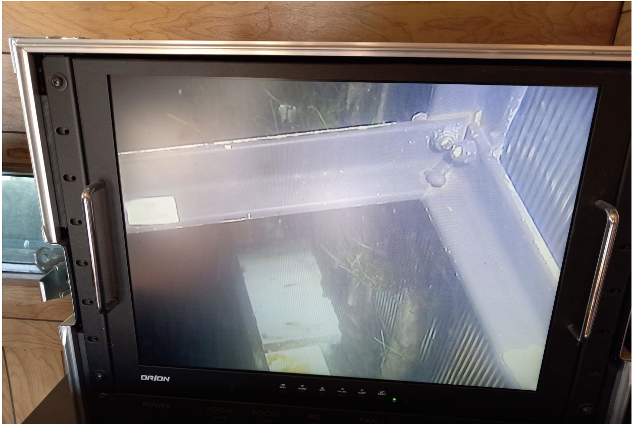
Photo 3: Debris on the brush bar and chain on ESBS in 1A slot.
