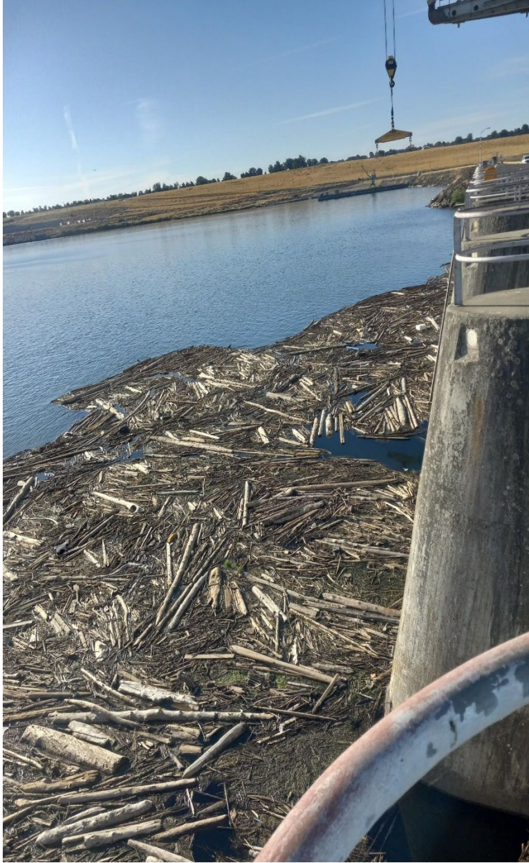
Photo 1: Forebay debris that had been in front of Unit 1 for a week to ten days.
