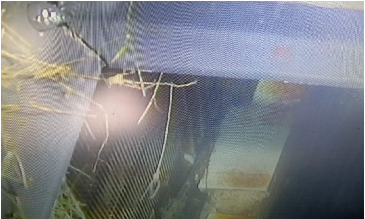
Photo 5: Debris on the brush bar and chain on the ESBS in 1B slot.
