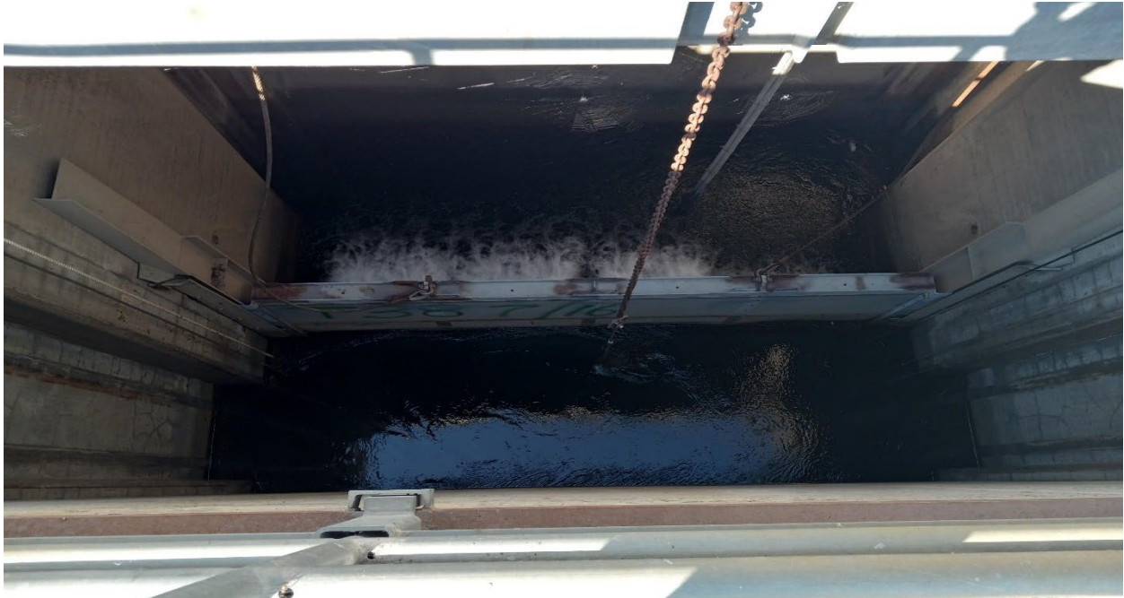
Photo 2: VBS differential caused by debris.
